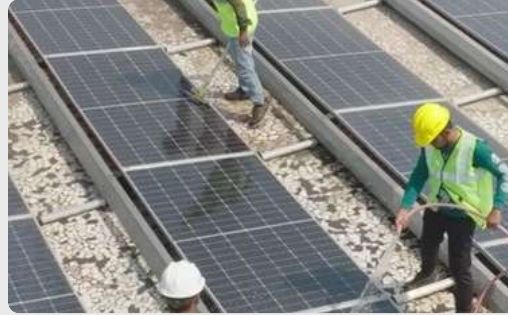
350kWp Solar Project at CST Technologies, Noida.
