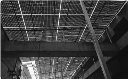
150kWp Solar Project at Bharti Realty, Gurgaon.
