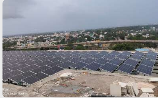
300kWp Solar Project at Income Tax Office, Bhopal.
