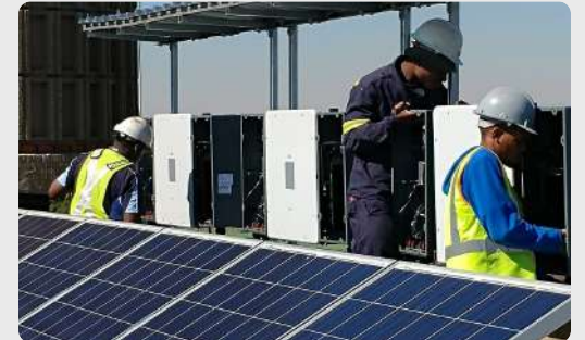
2MWp Operating Solar PV System at Panasonic, Jhajjar.
