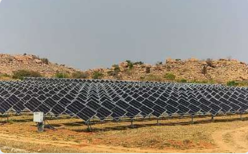
4.1MWp 2-axis Tracker Project for Greenko at Pavagada, Karnataka.
