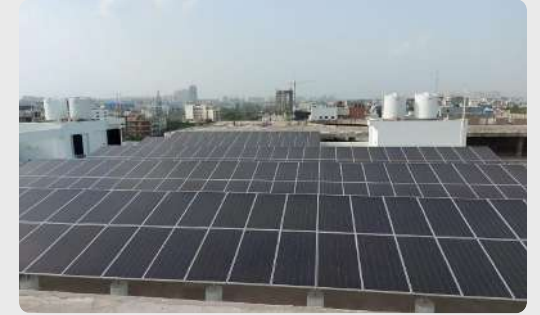
1.4MWp Solar Project Installed for Multiple Locations of Orient Fashion.
