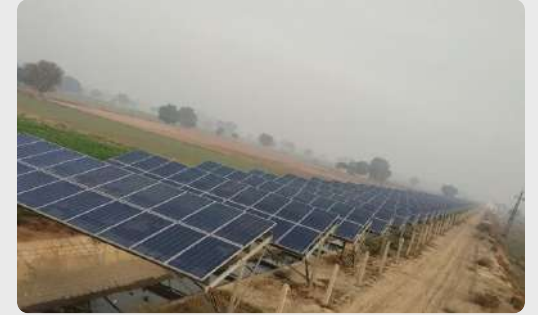
2.4MWp canal-top Solar Project for AGV Solar, Hanumangarh, Rajasthan.
