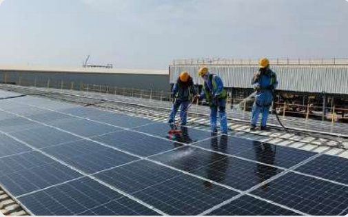
750kWp Solar Project at Roto Pumps, Noida.
