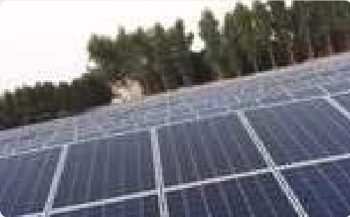
1.3MWp Solar Project for Sneha Farms c/o Tata International in Hyderabad.
