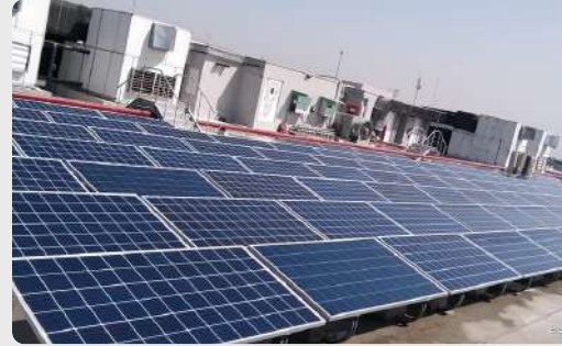
70kWp Solar Project at Supreme Court of India, Delhi.
