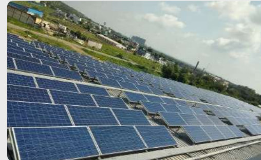
427kWp Solar Project at OK Play, Sohna.
