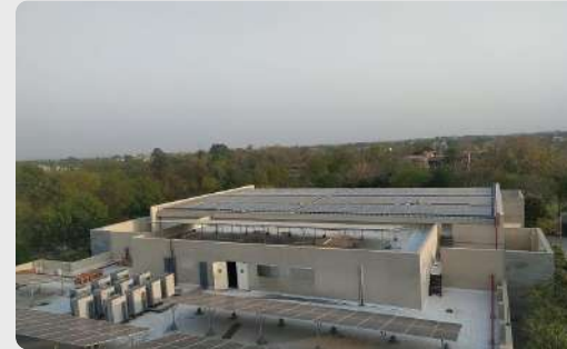
350kWp Solar Project at Courtyard by Marriott, Aravali Resort, Faridabad.
