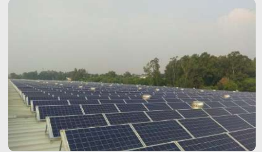
1.15MWp Solar Project for Godrej & Boyce Mfg. Co. at Mohali.
