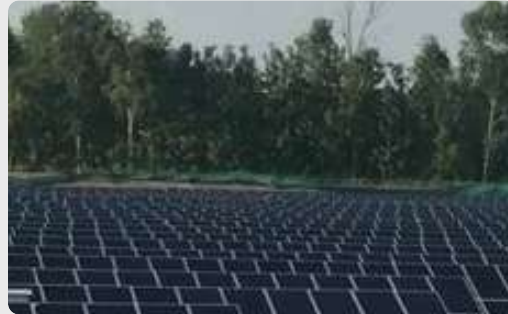
422kWp Solar Project for MES, Subroto Park, Delhi.
