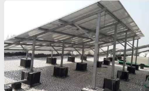
100kWp Solar Project at High-Rise Icon Towers, Gurgaon.
