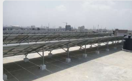
1.1MWp Solar Project for ESIC & EPFO c/o Avaada, Madhya Pradesh.
