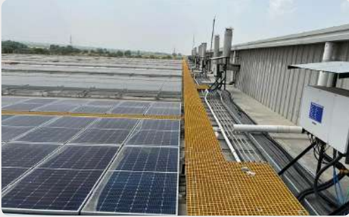
2MWp Solar Project at Denso, Jhajjar, Haryana.
