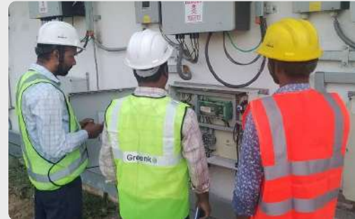
600kWp Operating Solar PV at Medanta, Gurgaon.
