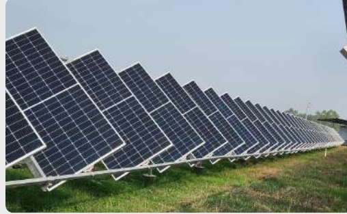
1.2MWp single/dual axis tracker Project for Advika Energies, UK
